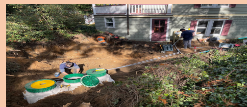
Fuji Clean CEN Series Installation in Sea Cliff, NY - Installation by Discount Cesspool.
